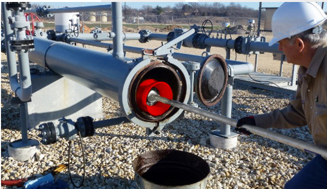
SAFE PIG RETRIEVAL IN FLAMMABLE GAS PIPELINES
